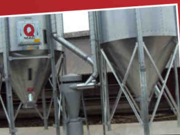
Dust cyclone fitted to 2 No. 150mm (6") exhaust pipes
