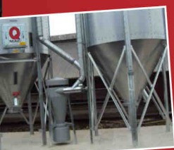
Dust cyclone fitted to 2 no 150mm (6") dia. exhaust pipes
